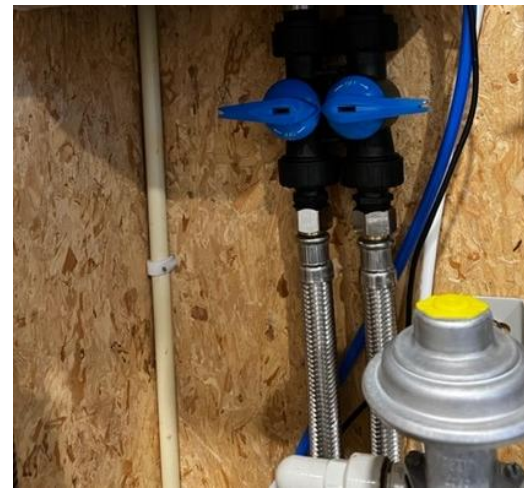
Bypass overdwars: Hard water
